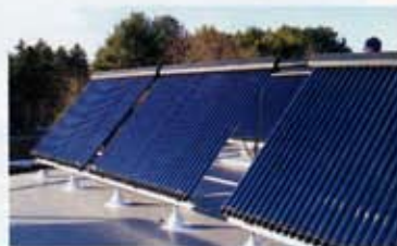
Evacuated tubes atop the Hilltop Lodge at OceanView, Falmouth, Maine.
