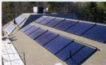
Workers installing solar thermal technology at the Cadigan Lodge in Topsham, Maine. Photo courtesy of Apricus.
